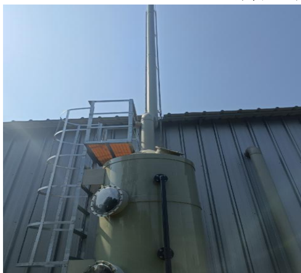
喷淋塔+排气筒
